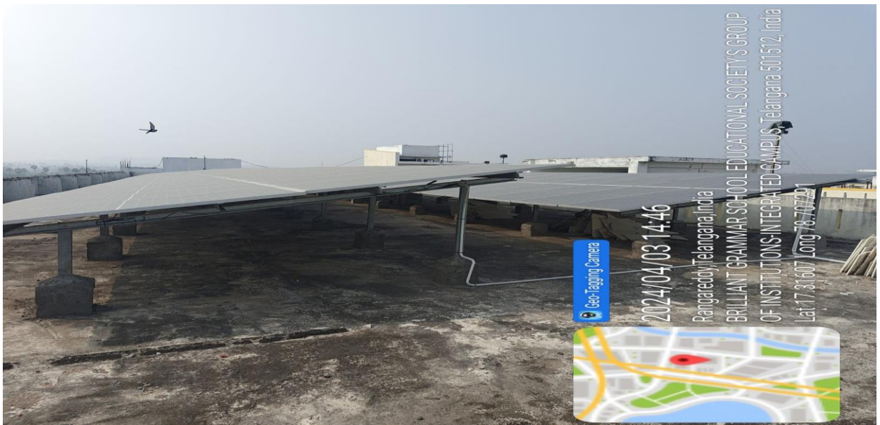
View of Solar Power plant 75 KWp.
